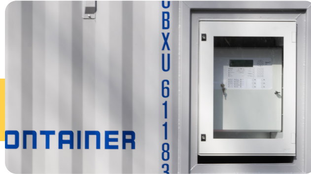
Integrated fire panel
