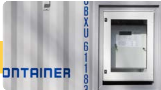
Integrated fire panel
